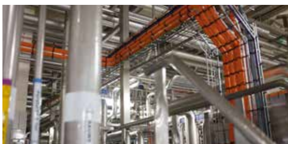
Operationalisation of the second part of the facility for the production of milk powder and infant nutrition at FrieslandCampina Ingredients in Borculo (Netherlands).
